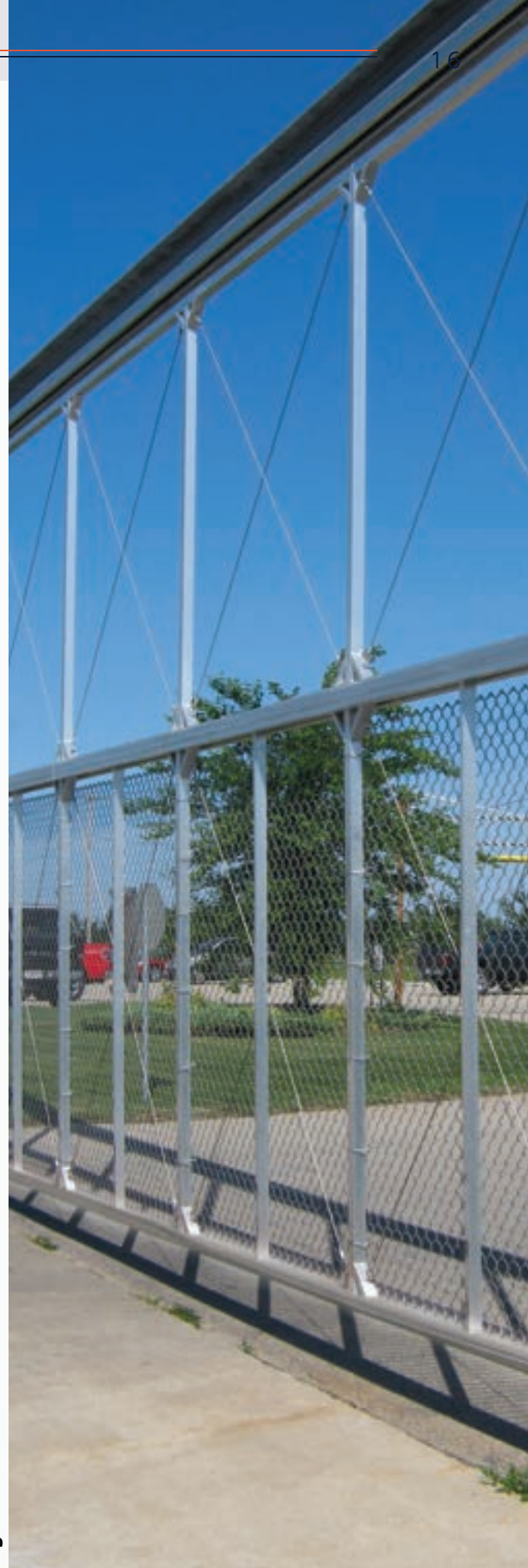
Right: Overhead Slide Gate.
