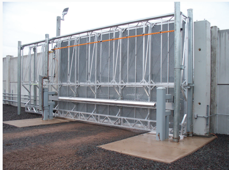
Right: PPL Electric Utilities, TCGR-12.
