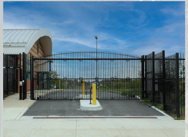
Right: Structural Cantilever Slide Gate.
