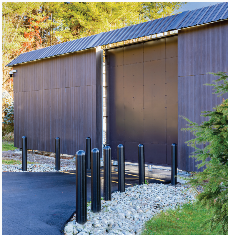
Right: Eversource Sharon Substation, Custom Structural Cantilever Gate. Pg. 14
